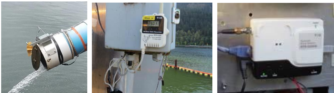
Figure 3. Mechanical counter components used to enumerate lamprey passage at Bradford Island AWS and Cascades Island Entrance including the limit switch attached to exit paddle and cushion, wireless data recorder, and network base station (from left to right at BI-AWS LPS).
