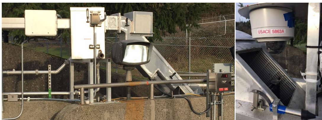
Figure 5. WA-AWS LPS exit showing (left to right) PIT antenna, upwelling box with black latch, camera box & paddle, and Dwyer counter display with red warning tags. Right panel shows camera box with lid removed, globe camera, and proximity detector with blue tape pointed at curved metal tab indicating position of paddle (open/closed).
